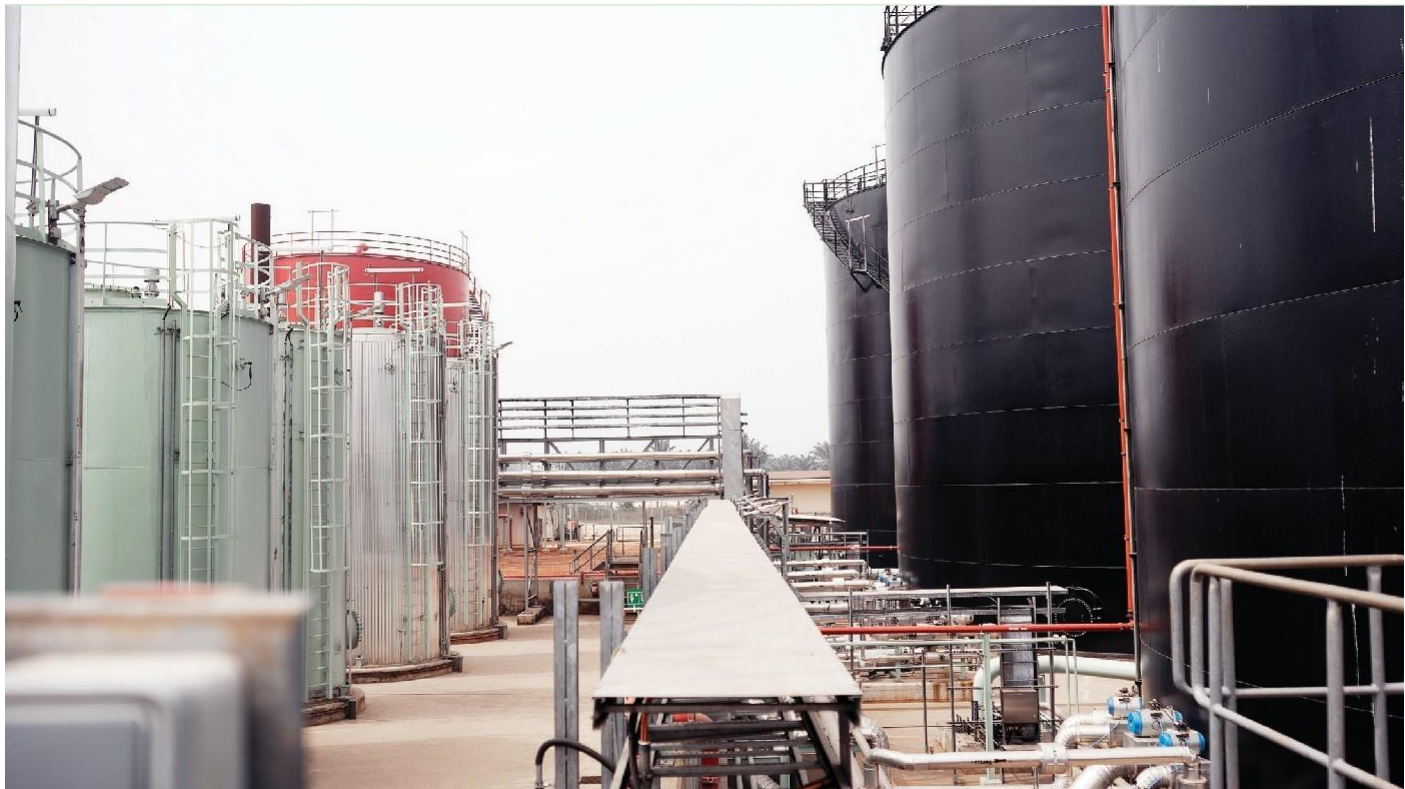
The MARIA GLETA project, which is partially funded by EBID is a thermal power station in Benin.
