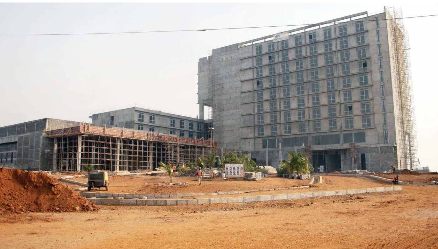
Cape Sierra Hotel Construction Project - Freetown, Sierra Leone. Co-financed by the Bank
